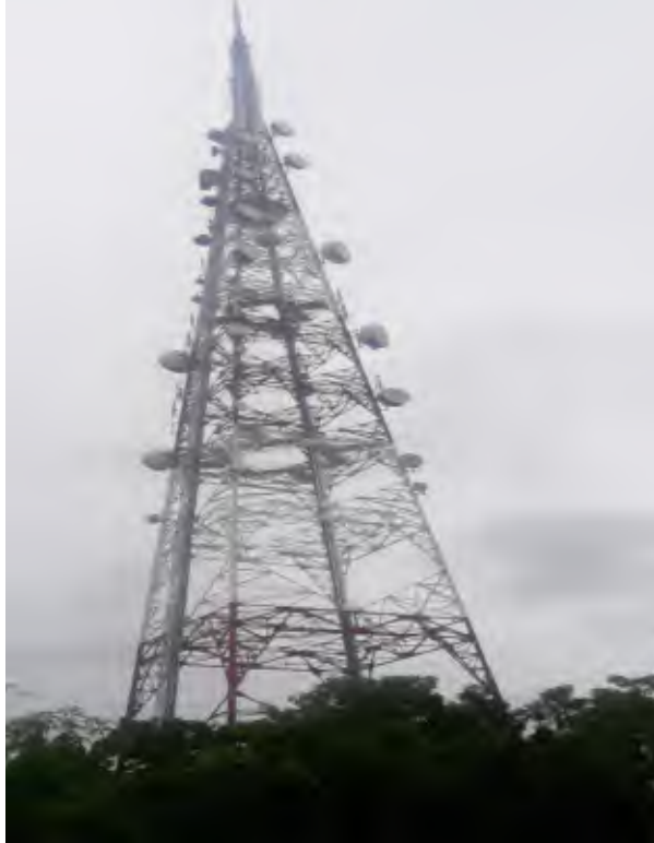
Kokavil communication tower
